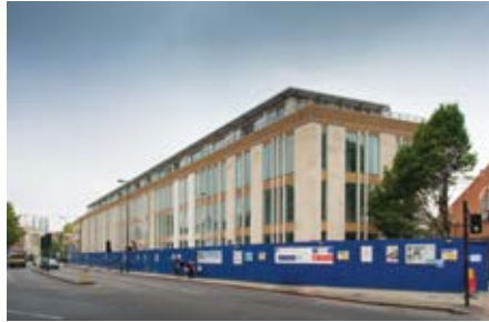
Project : Edinburgh House, London Contractor : Sapphire Mechanical & Electrical Services Location : London, England Year : 2018
